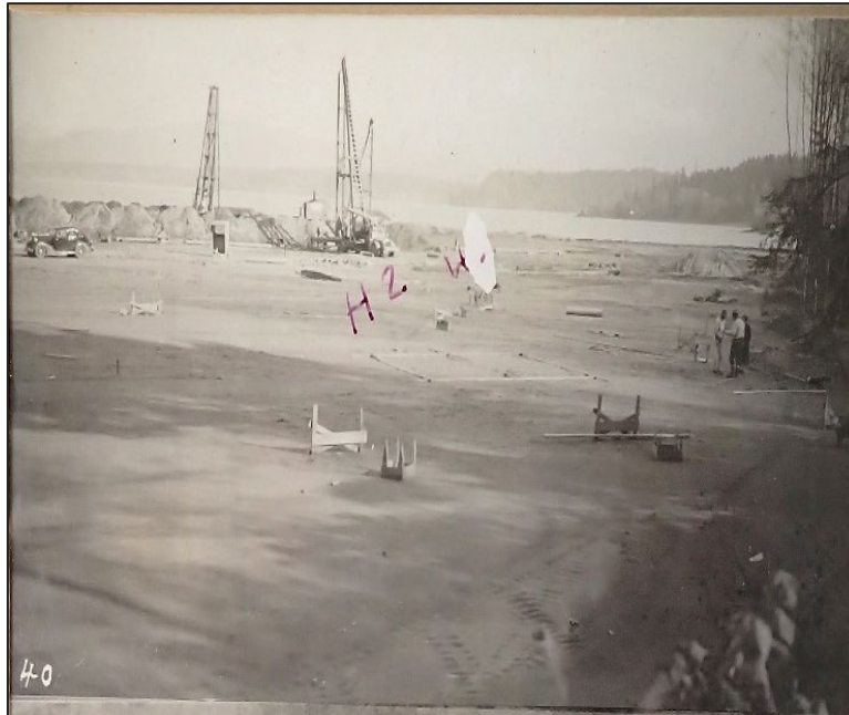
Photograph 2. Pile driving, April 1940 (Photo on file at DOL; markings on photo are on original)
