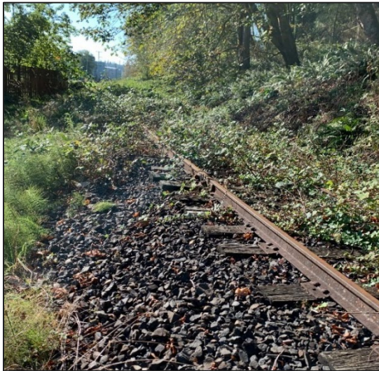
Photograph 8. Dormant spur, looking south (Photo by Tetra Tech, 10/5/20)
